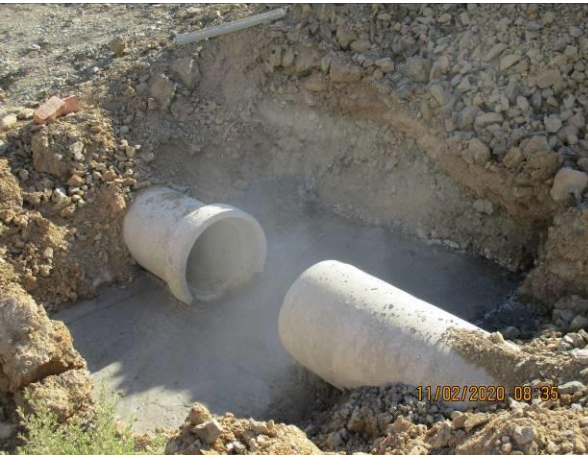
Photo: Manhole for storm water drainage.
